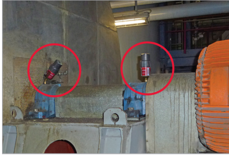
Industry: Waste incineration plant
