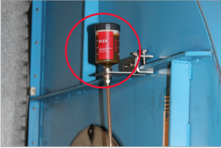
Industry: Waste incineration plant
