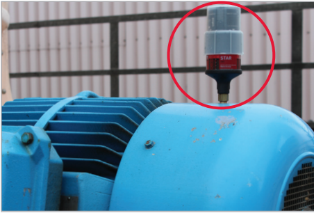
Industry: Power Generation
