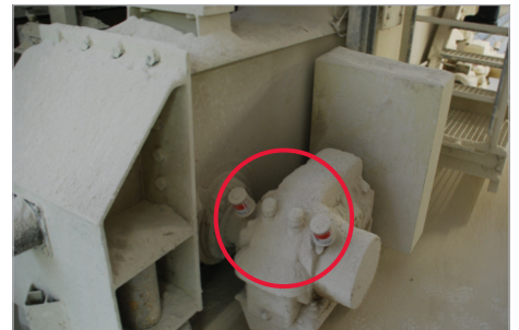
Lubrication on mixer shaft
