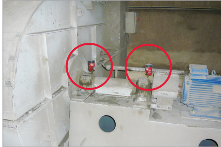
Lubrication of pillow block bearing on a fan shaft
