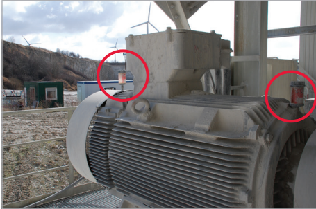
Lubrication of motor on a vibrating screen
