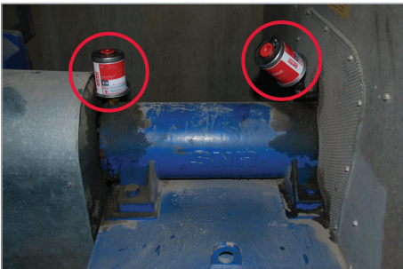
Lubrication of pillow block on fan
