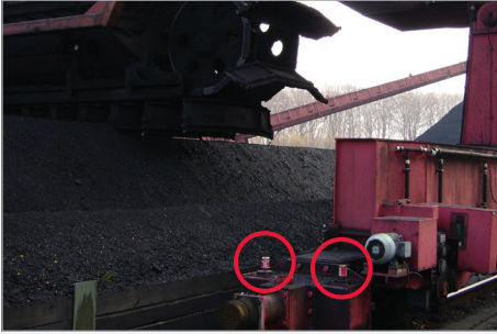
Lubrication of flange bearing on support rollers
