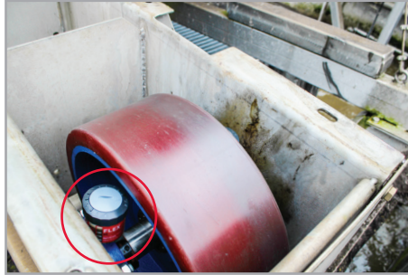
Grit and grease removal: Lubrication of flanged housing units at the scraper
