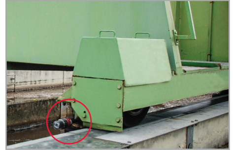
Primary sedimentation tank: Lubrication of impeller wheel bearing
