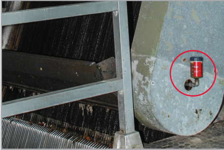
Screening: Lubrication of chain guide rollers
