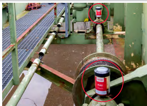
Roller bearing lubrication on a scraper
