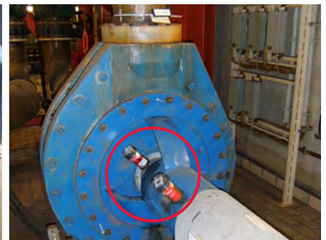
Drive shaft lubrication on a pump
