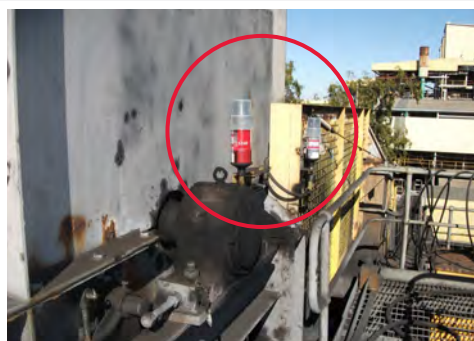
Lubrication systems on a conveyor
