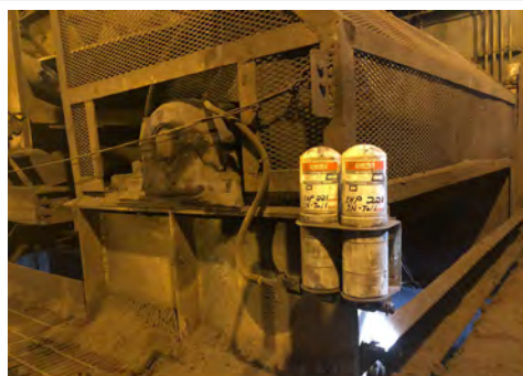
Lubrication on a conveyor
