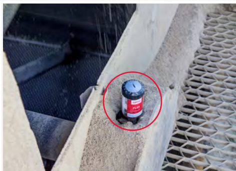
Lubrication of pillow block bearing on grit and sand screen
