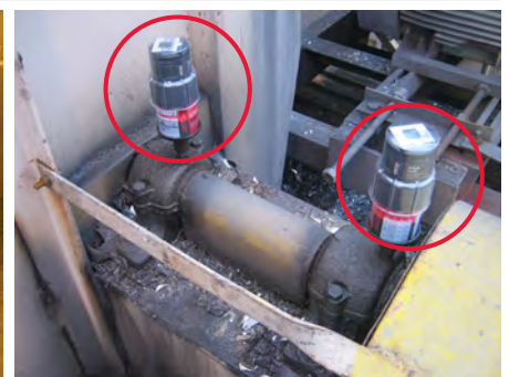
Lubrication of a fan drive shaft bearing
