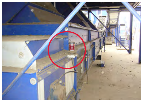
Flange bearing lubrication on a conveyor
