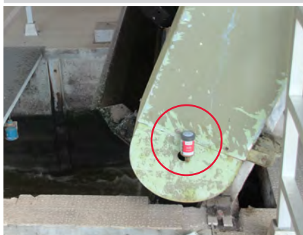
Roller bearing lubrication on a chain guide roller
