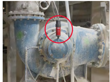
Bearing lubrication on a pump
