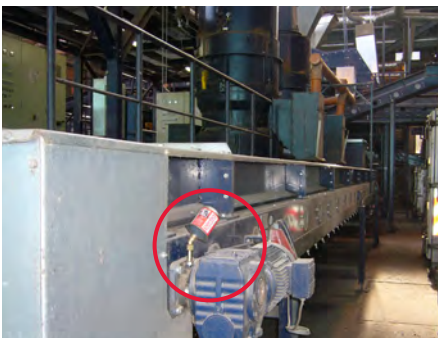
Flange bearing lubrication on a conveyor
